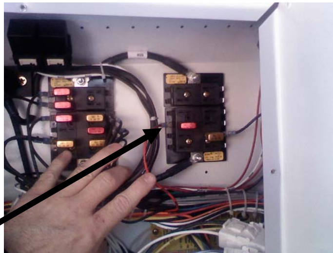
Example: 2502B And 10 Amp Breaker Connected to Ignition Powered Position.
